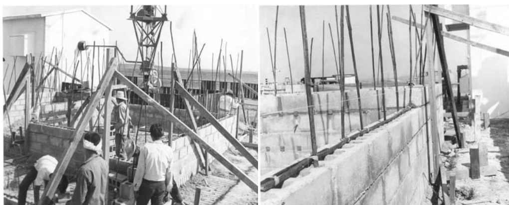
Figure 3- 17 Bamboo reinforcing being used in concrete block construction by the US Navy for a radar site at Tarlue Naval Station in the Philippines
